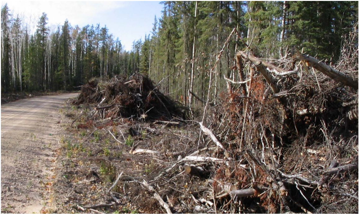
Figure 3.6 Roadside right-of-way construction. The removal of adjacent forest permits regular maintenance activities.
